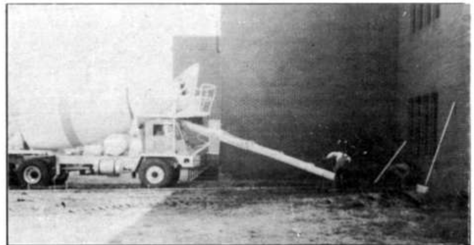
Construction workers pouring a new concrete sidewalk, one of the many renovations going on at LOHS.
