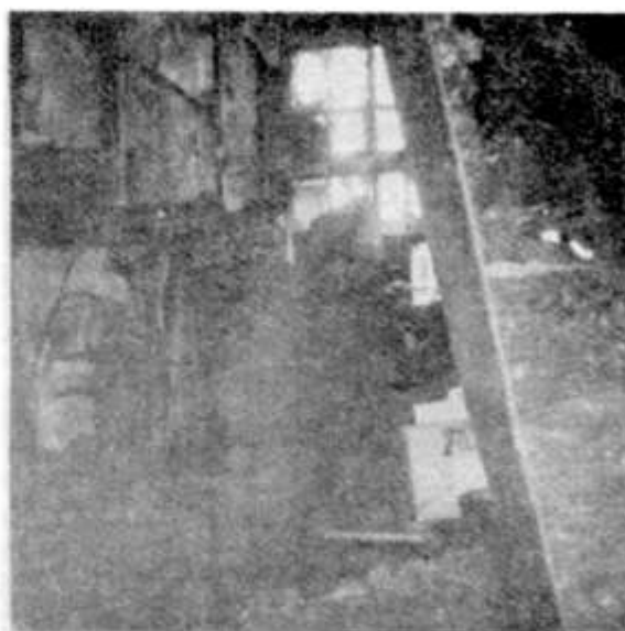
PORTIONS OF ROOF which fell in on the Journalism Room.
